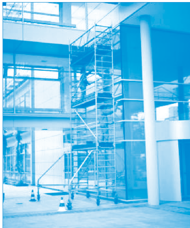
Example 3: Cleaning glass atria and roofs from the inside using a mobile elevated work platform (MEWP) – scissor or a vertical telescopic lift
