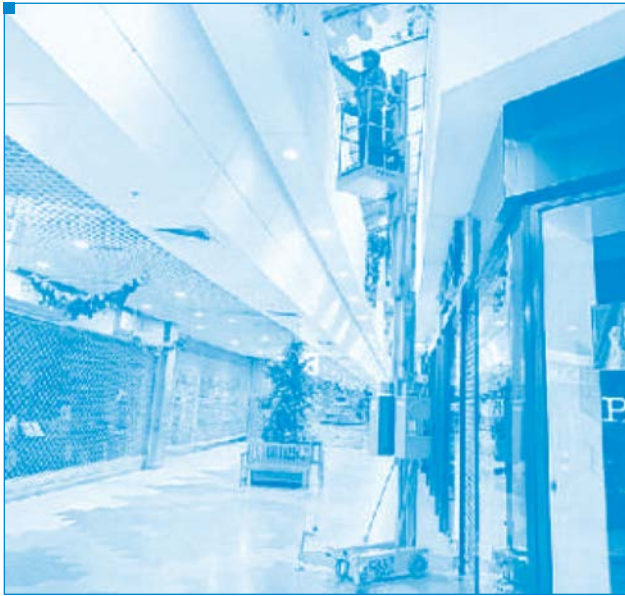
Example 4: Cleaning glass atria and roofs from the inside using a mobile elevated work platform (MEWP) with boom
