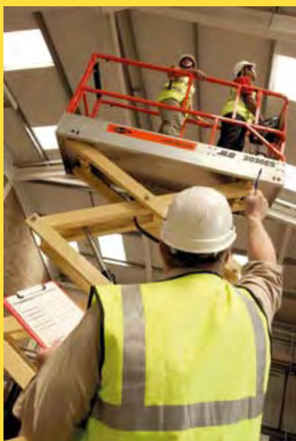
Training makes operators aware of potential dangers and the safety measures needed to overcome these risks.
